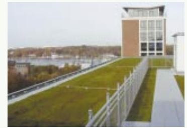
This lightweight roof is used as an outdoor terrace by occupants of the Family Services of the Rostock building in Germany.
