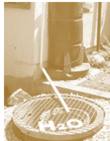
RAINWATER COLLECTION SYSTEM
